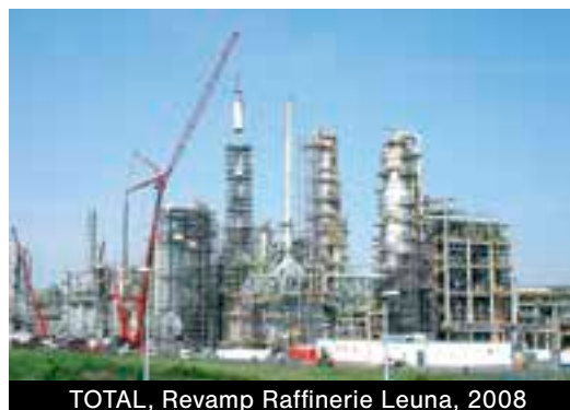
TOTAL, Revamp Raffinerie Leuna, 2008
