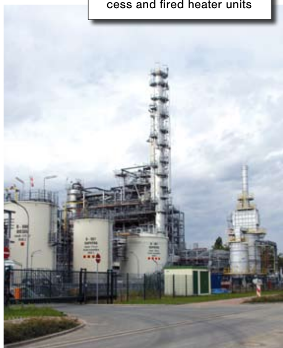
Partial view of the Hylube2 plant with product tanks, process and fired heater units
