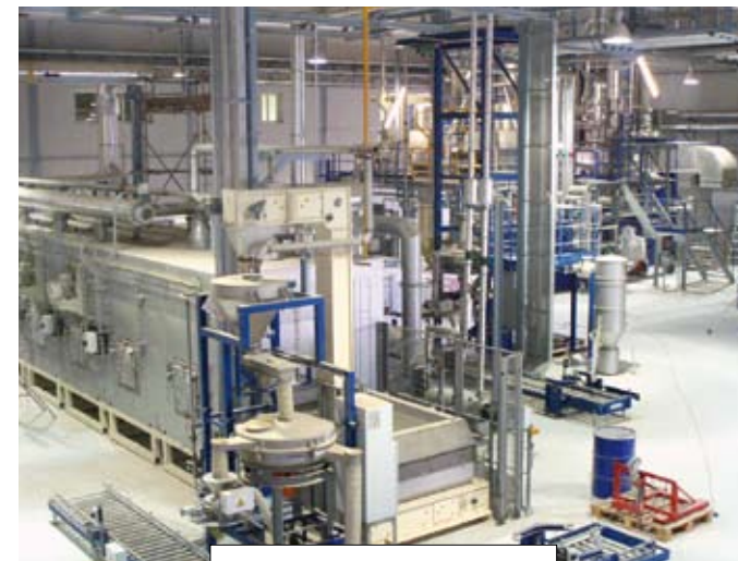
Interior view of the plant
