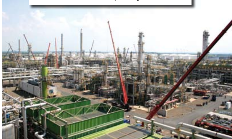
View over TOTAL Refinery during the shutdown
