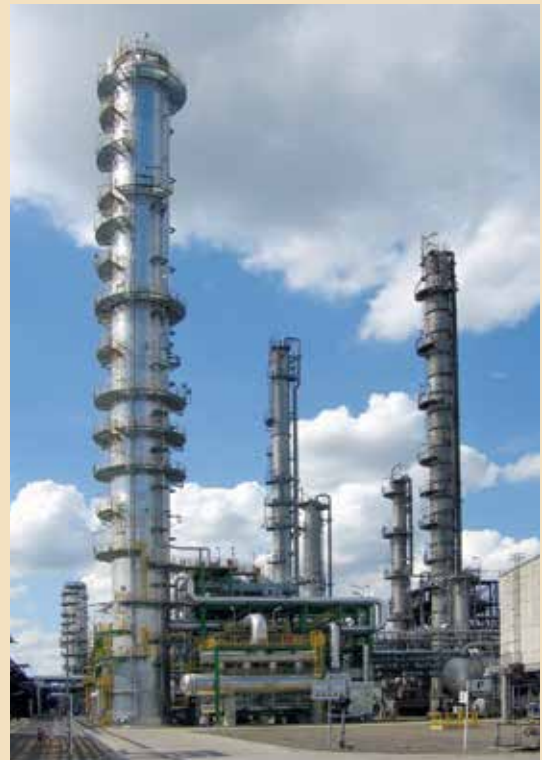
C 3 splitter at PCK Schwedt, Germany, with vapour compression, reboiler/condenser, equipped with UOP HIGHFLUX tubes
