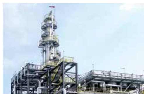
HDS1 plant at OMV Refinery Schwechat, Austria
