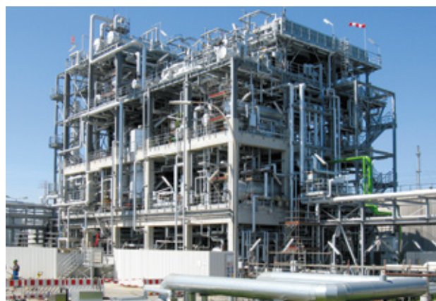
Fig. 2: Propane deasphalting plant (PDA), H&R Ölwerke Schindler GmbH, Hamburg, Germany
